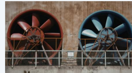
Energy Service / Power & HVAC Systems
