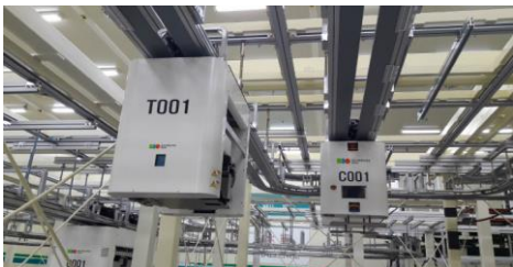
Overhead Hoist Transport
