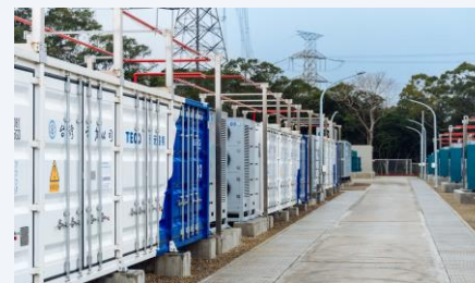
Energy Storage EPC
