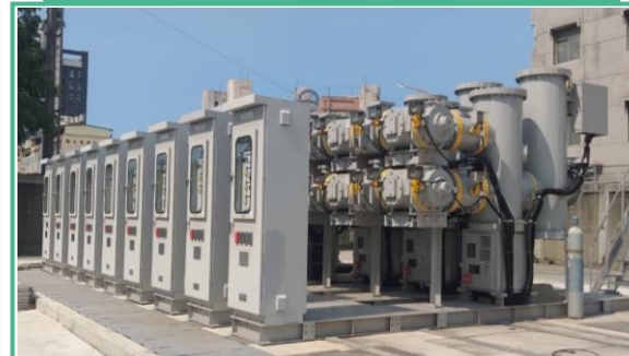
Taipower Distribution Substation
