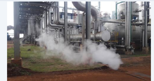
Waste Heat Recovery
