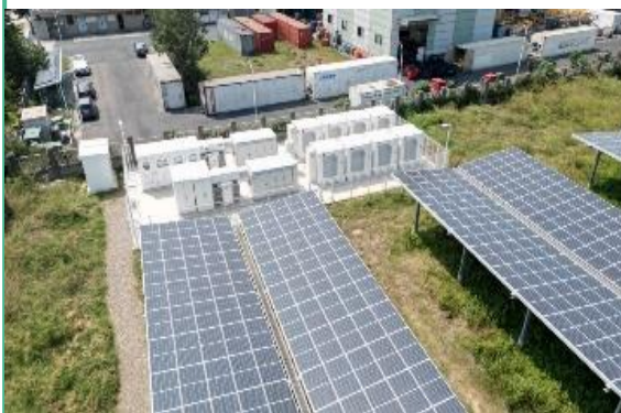
Taoyuan 2+4MW/2+4MWh AFC Energy Storage System
