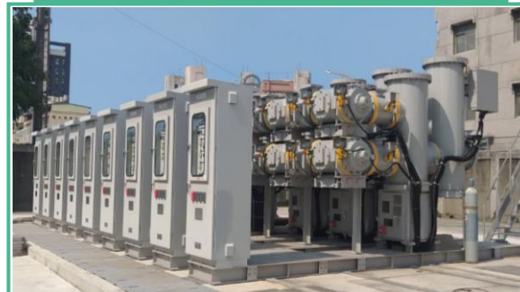
Taipower Distribution Substation
