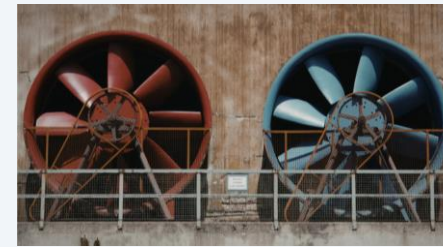
Energy Service / Power & HVAC Systems
