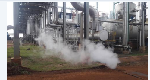
Waste Heat Recovery
