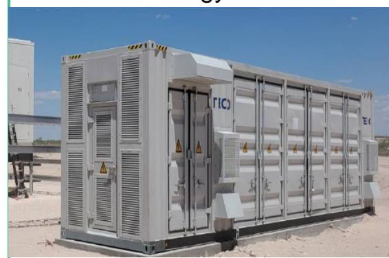
US 2MW/2MWh Energy Storage System Frequency Regulation Service
